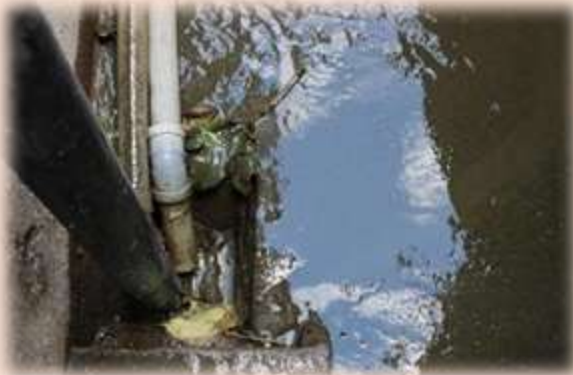
It turned out that the TW team had flushed the sewer, and all the muck – thick, black, greasy gunk – came to our gulley.
